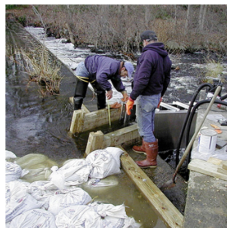
A crew from NOAA installs a ladder on a dam in Massachusetts.
