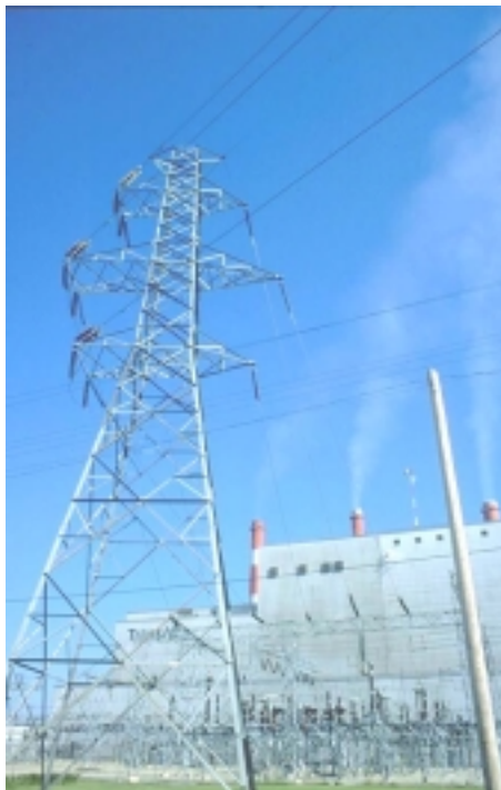
Electricity is produced at large power generating stations and carried to customers over long distances by a system of overhead power lines.
