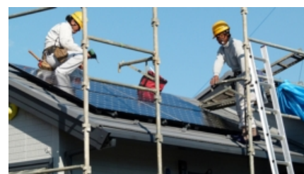
Solar power installation in Japan. Credit: CoCreatr via flickr
