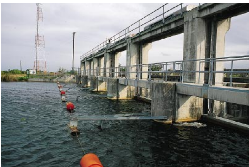
FOUR WATER-CONTROL GATES, including this one, punctuate the Tamiami Trail, which runs across southern Florida from east to west. The gates regulate the amount of water that flows south into Everglades National Park.
