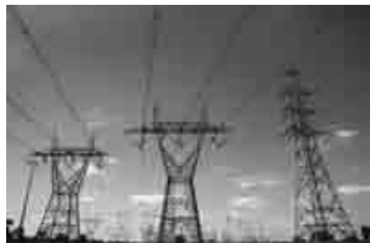
Transmission lines carry electricity at high voltages over long distances.
